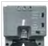
Inner control panel
